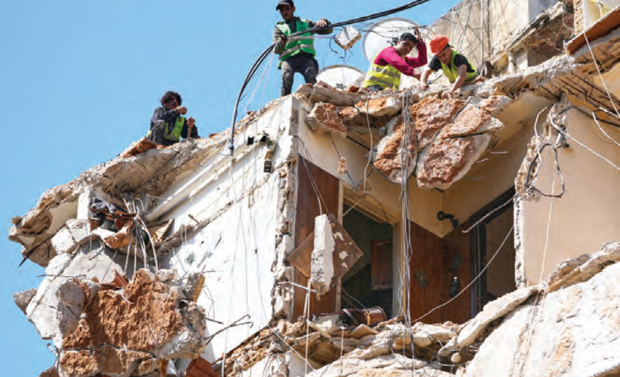
Workers remove the rubble as rescuers keep searching for a missing woman and girl at a destroyed building that was hit on April 8, in an Israeli airstrike in Beirut, Lebanon
