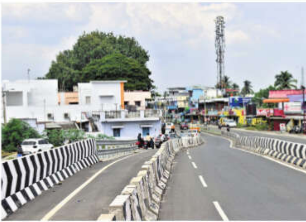
After the flyover was completed in December 2023, it soon drew criticism for multiple design and engineering flaws | FILE PIC
