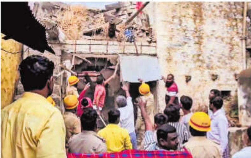
Rescue personnel clear debris after a house roof collapsed during heavy rain and strong winds, killing four members of a family, in Vijayapura, Karnataka, Friday (PTI)
