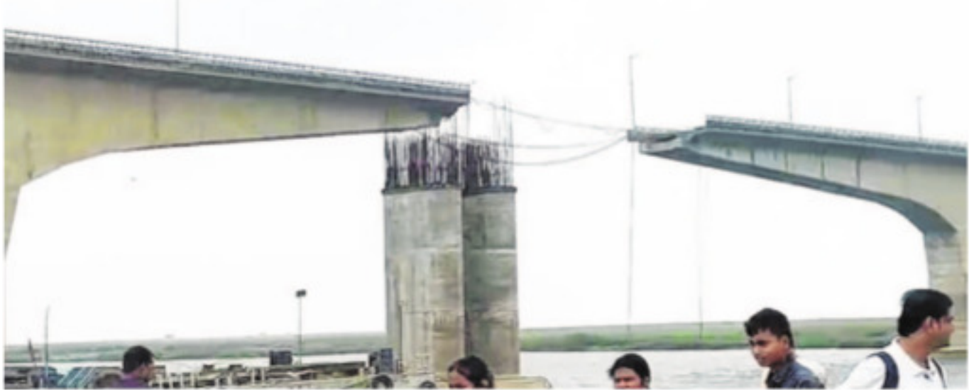
A slab of the Vikramshila Setu bridge (near pillar 133) collapses into the Ganga River in the early morning, in Bhagalpur
