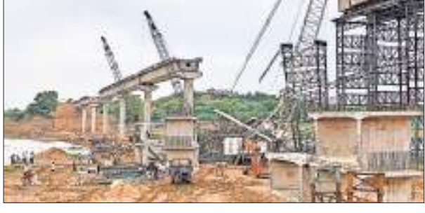
Officials at the site of the bridge collapse, which left six labourers dead and three injured, in Hamirpur district, Uttar Pradesh. FILE
