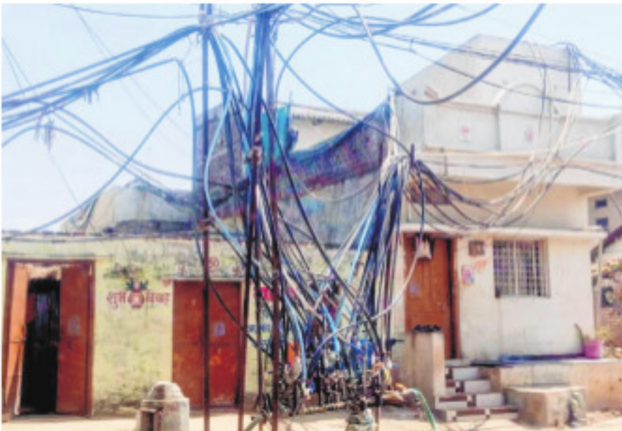
Multiple pipelines connected to a single borewell expose severe water supply mismanagement.
