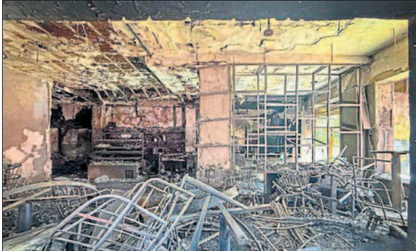
21 people had died in a fire at an illegally run B&B facility in Hauz Rani in Delhi on June 3.
