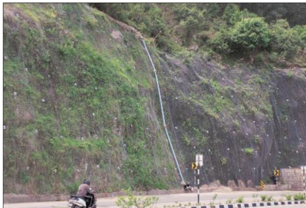
The drainage pipe network on Kaithlighat-Kandaghat section of the Kalka-Shimla national highway. SAURABH PARASHAR
