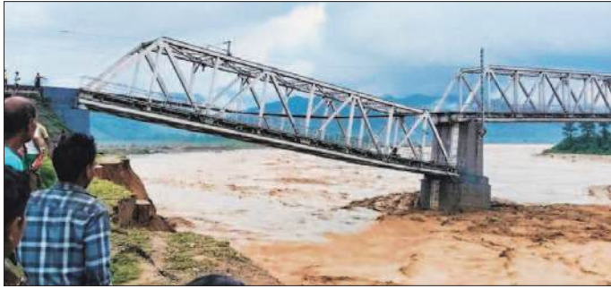
A railway bridge tilts after severe bank erosion caused by heavy rainfall between Archipathar and Simen Chapari stations, in Dhemaji district, Assam on Monday. (PTI)
