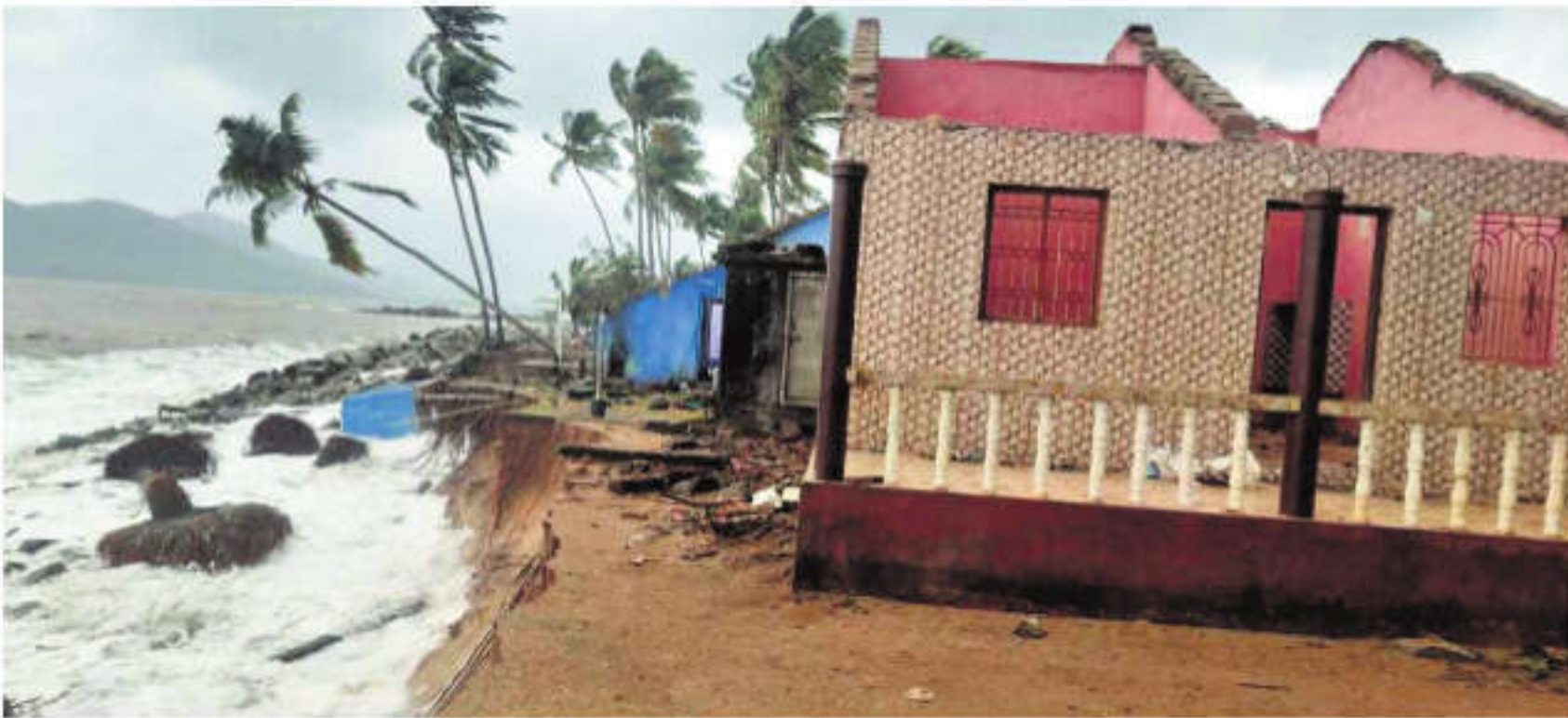
A damaged house which was abandoned by a resident of Harwada due to sea erosion | EXPRESS
