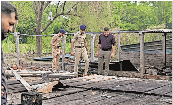
Rescue efforts underway after the explosion at the firecracker unit in Ramol area of Ahmedabad on Saturday. BHUPENDRA RANA
