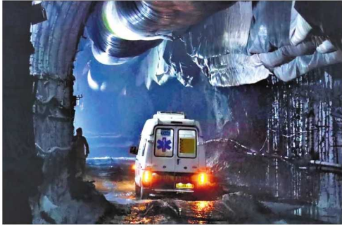
The tunnel collapsed following an explosion suspected to have been caused by methane gas.
