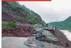
A portion of Jammu-Srinagar National Highway damaged at Udhampur.
