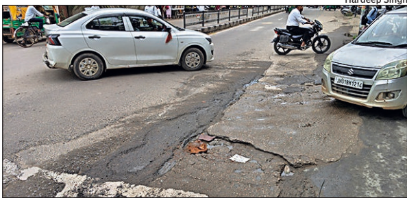
The first identified stretch is the 7.9-km corridor from LPN Sahdeo Chowk to Booty More, which has suffered extensive surface erosion
