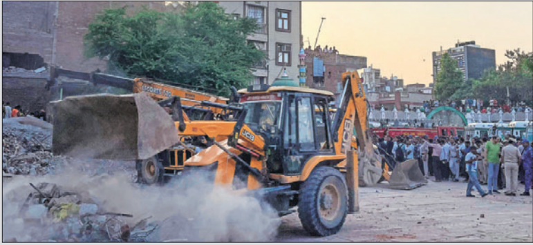
An earthmover clears debris after a four-storey building collapsed onto two to three adjoining houses, in Seemapuri, New Delhi, on Wednesday. (PTI)
